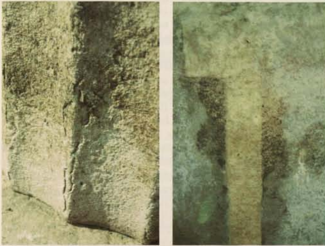
Fig. 14a-b. Milet, marble columns: Surficial carbonate precipitation mainly caused by the metabolic activity of photosynthetic algae and cyanobacteria (a) and different cleaning treatments (laser, mechanical and chemical procedures) to remove the aesthetical detrimental crusts (b).
