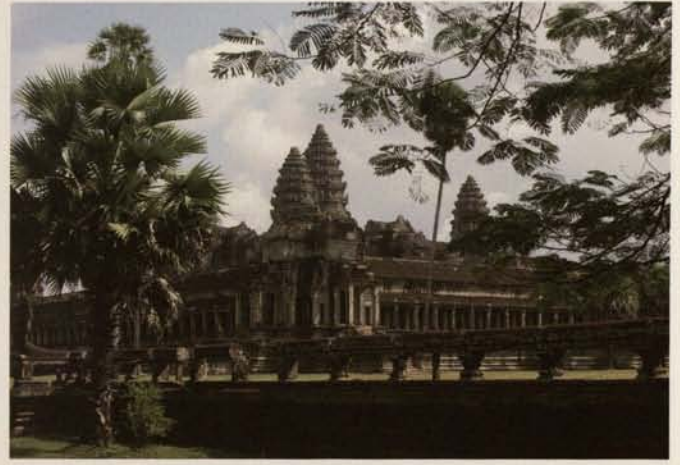
Fig. 8. Angkor Vat, temple: Natural stone affected by biocorrosive and biofouling microorganisms.
